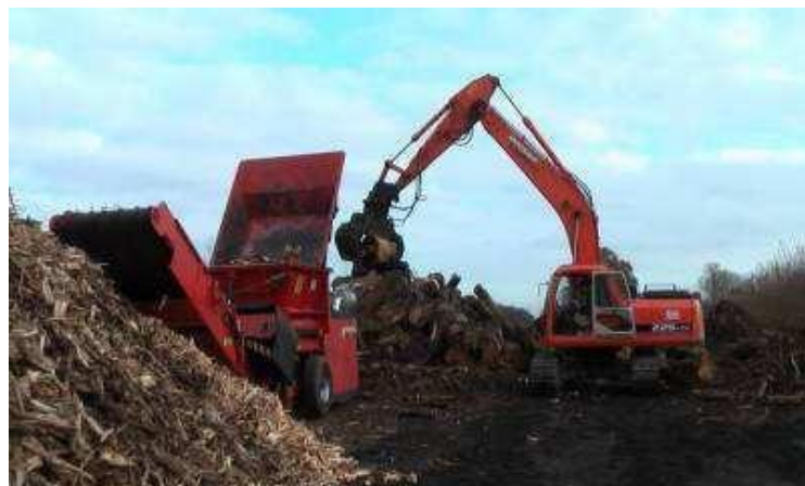
Wood pre-treatment and storage plant.
